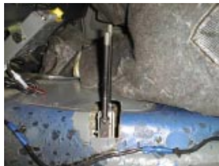
A new hole must be cut into your floorboard to fit the new handle assembly.
