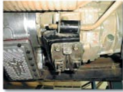
The modified transmission bracket with the rubber support in the new location.
